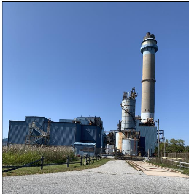
Figure 1 – Air Scrubbers and Buildings
